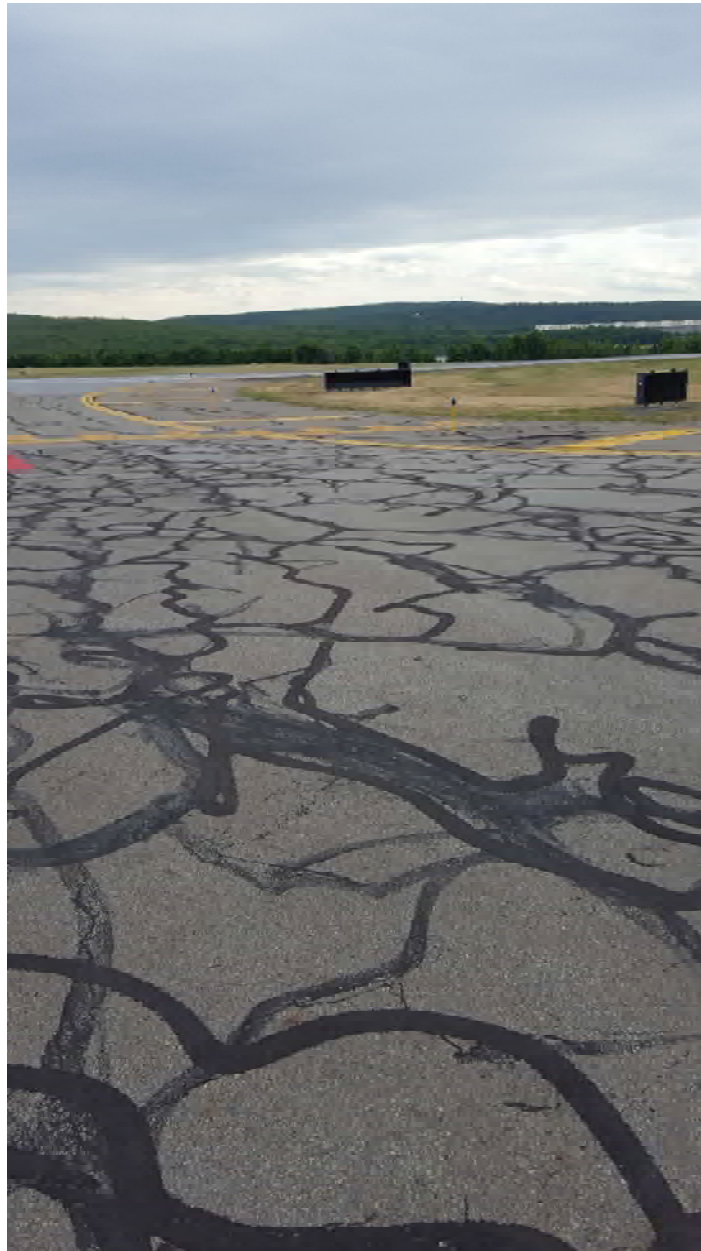
Taxiway C Medium Block Cracking
