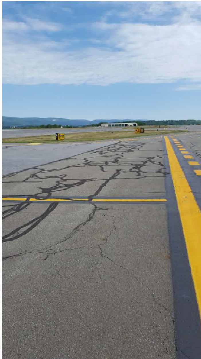
Taxiway B3 Low Block Cracking
